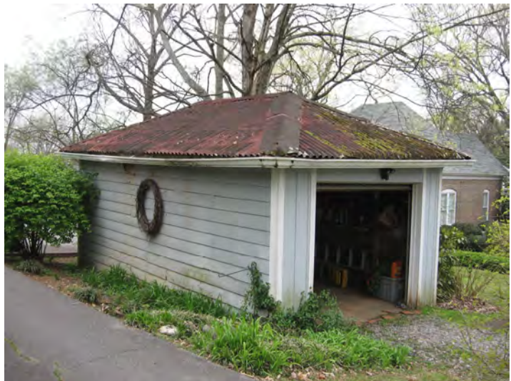
This single bay garage retains much of its original design (507 N. Ingleside Avenue).
