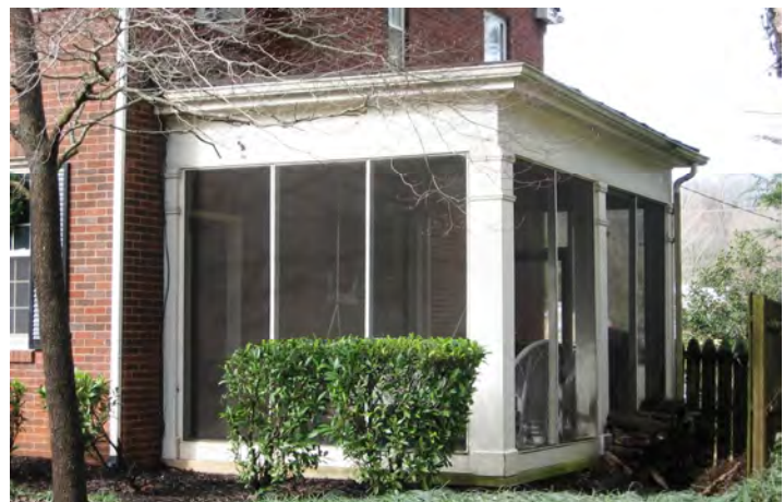
The side porch at 708 Ingleside Avenue is an appropriate example of screen panels.
