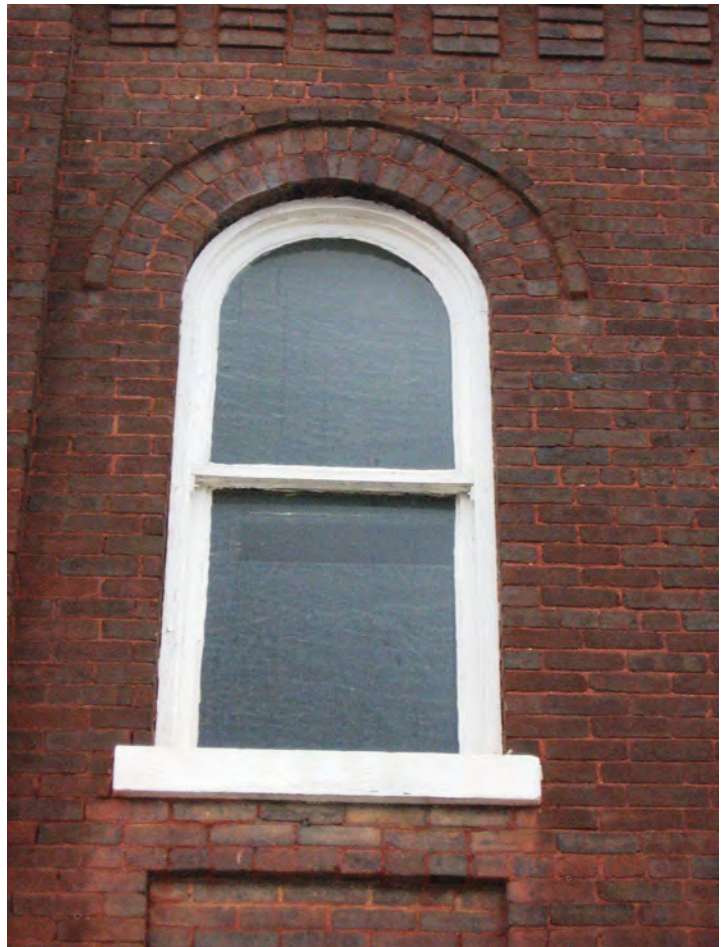
Retain original windows such as this arched, one-over-one, wood-sash example at 10 N. White Street.
