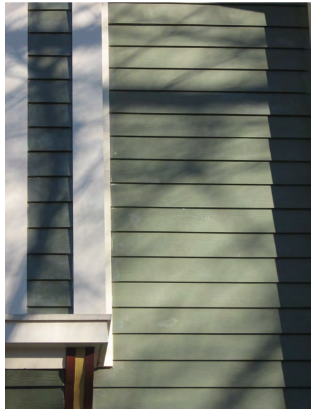
Cementitious siding may be appropriate to replace deteriorated siding or for new construction.
