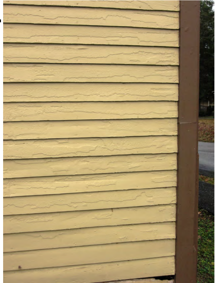
Original wood siding is important to a dwelling's historical appearance and should be maintained (510 E. Madison Avenue).
