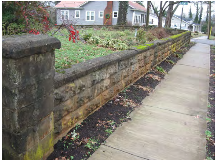
It is important to preserve and maintain original retaining walls of stone, brick or rock-faced concrete block such as this wall at 616 E. Madison Avenue.
