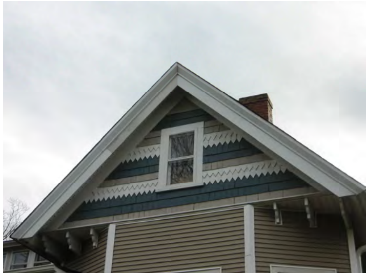
Exterior wood siding requires thorough scraping and priming prior to painting (615 Ingleside Avenue).
