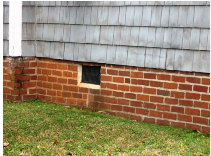
Brick foundations should be repointed with brick and mortar to match the original (7 Atlantic Street).
