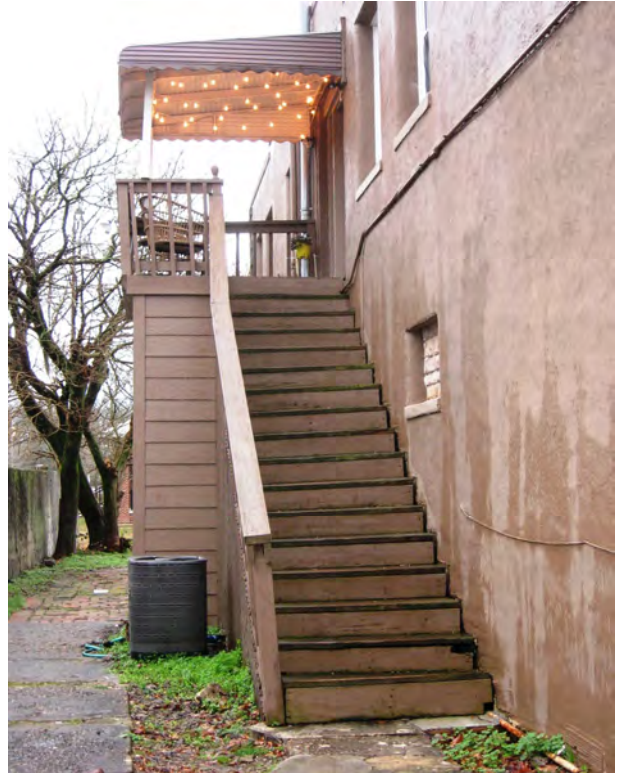
Locate fire escapes and staircases on side or rear elevations (113-115 E. Madison Avenue).
