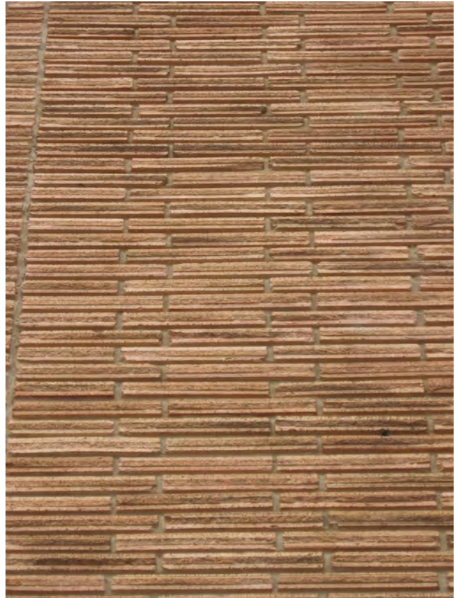
Historic masonry surfaces include materials from the 1950s and 1960s such as the “Roman Brick” at 16 N. White Street.
