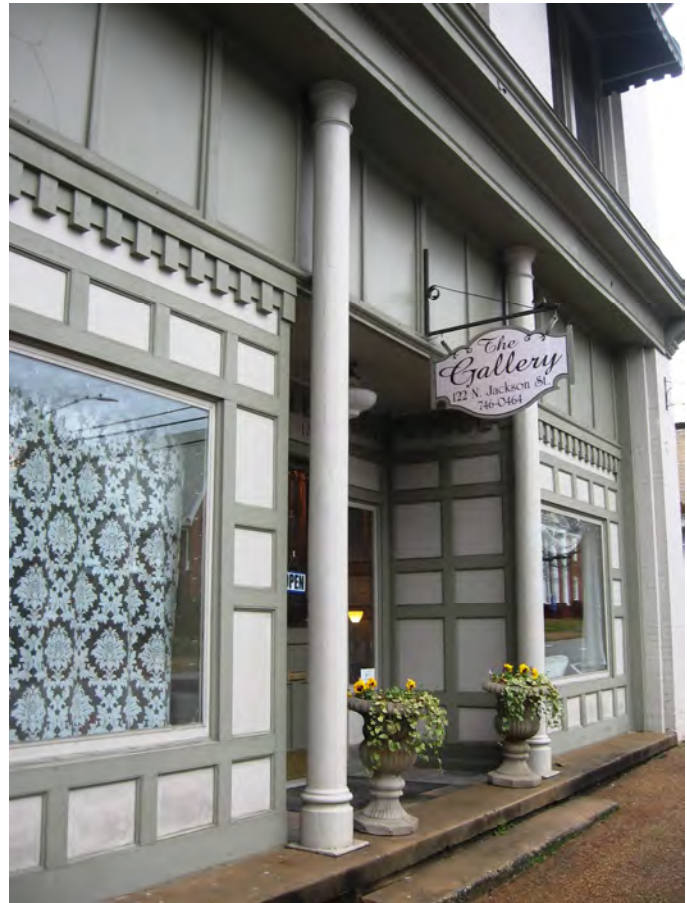
Cast iron was a popular feature on commercial buildings of the late 19th century, as seen at 122 N. Jackson Street.
