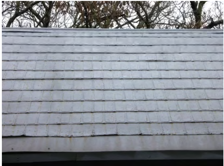
The dwelling at 500 E. Madison Avenue retains its original pressed metal roof. These types of roofs should be repaired and retained.
