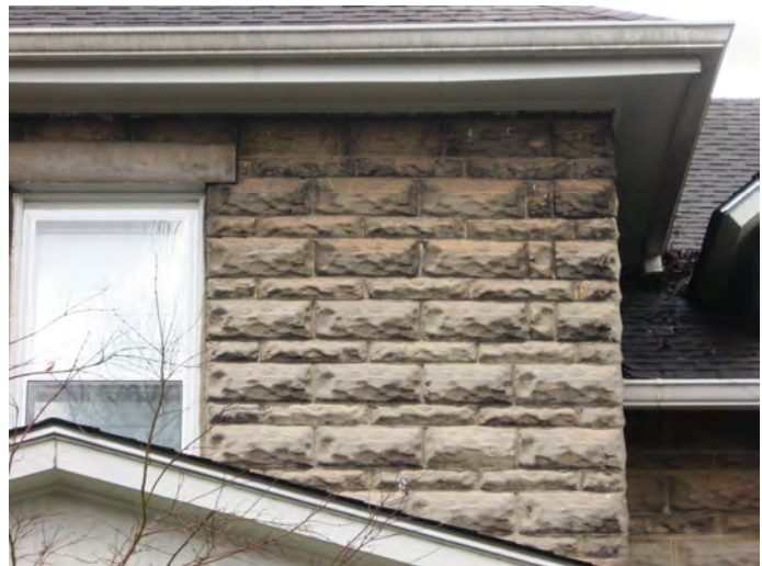
Keep masonry surfaces, including rock-faced concrete block, in good repair (616 E. Madison Avenue).
