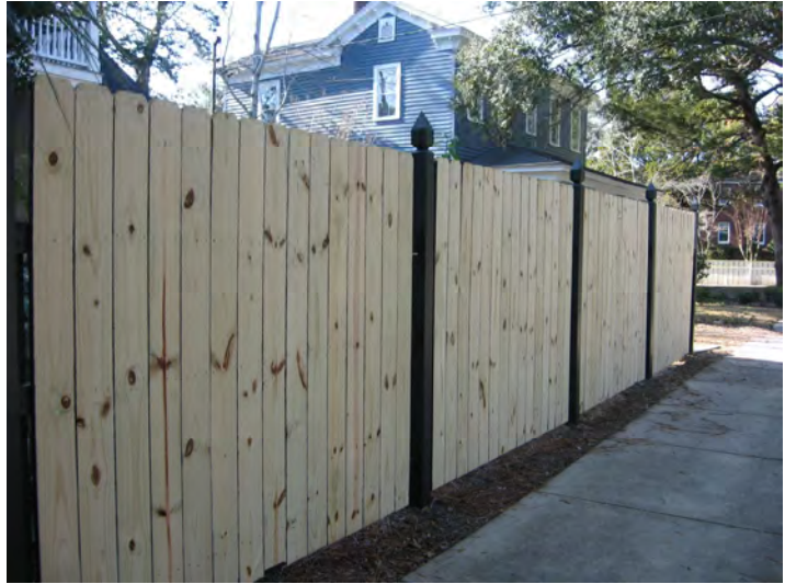
Privacy fences should be designed to have the structural support system on the inside of the fence and not the outside as in this example.
