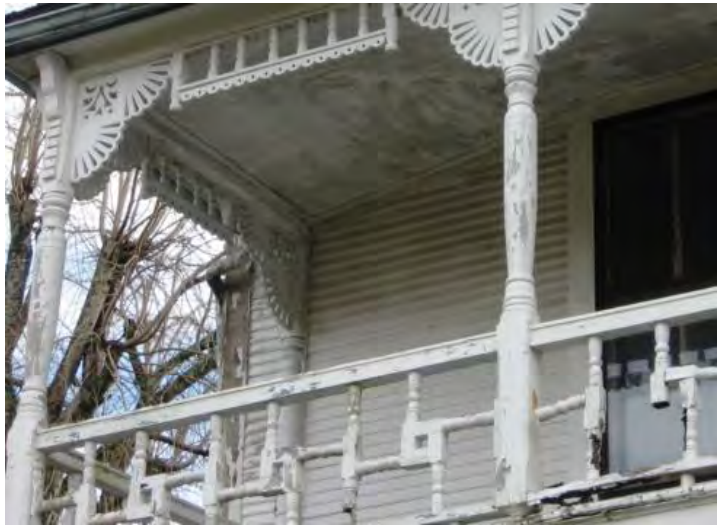
Replace only the missing pieces of a porch feature, such as the missing segments of this unique porch railing, rather than the entire railing (501 E. Madison Avenue).
