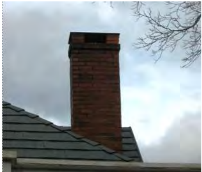
A number of dwellings retain original brick chimneys that require regular inspection of flashing where adjoining the roof (418 E. Madison Avenue).
