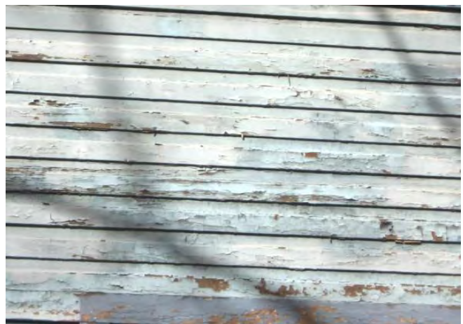
Blistered paint layers should be removed to the next intact layer, which may be the bare wood surface.
