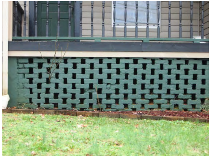
A pierced brick foundation like the one at 607 Ingleside Avenue should be maintained and kept visible. Do not cover, conceal, or infill this historic feature.
