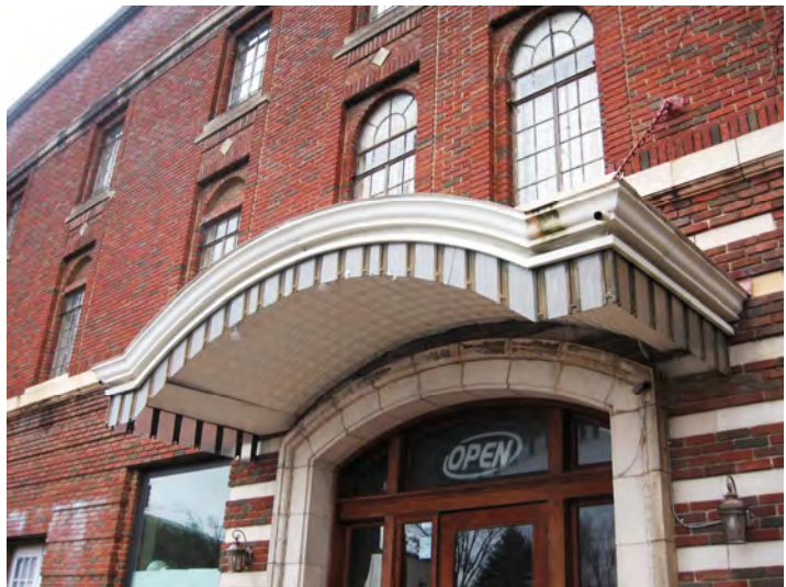
The metal canopy over the entrance at 3 N. Jackson Street is a significant façade feature that should be preserved.
