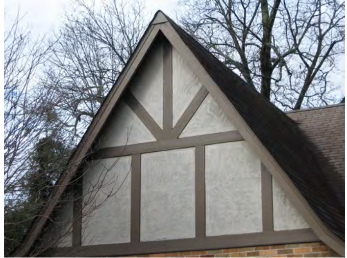
The use of stucco may be a character-defining detail in Tudor Revival-style dwellings (612 Ingleside Avenue).
