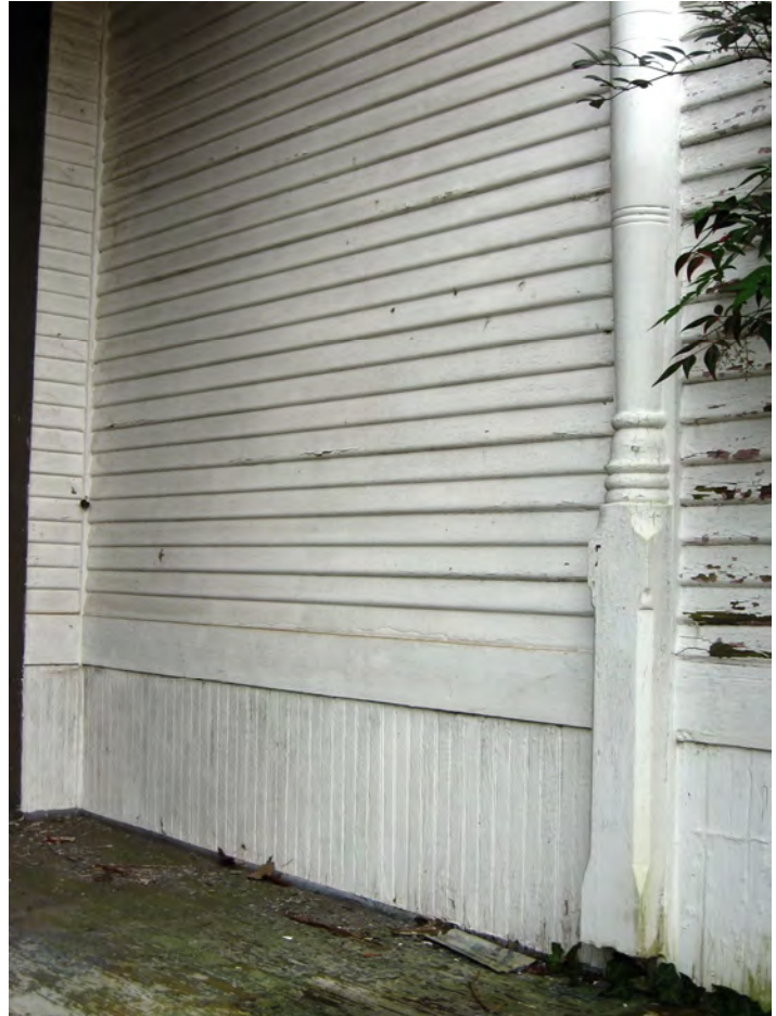
Preserve and maintain original wood siding through proper painting and regular maintenance (505 E. Madison Avenue).
