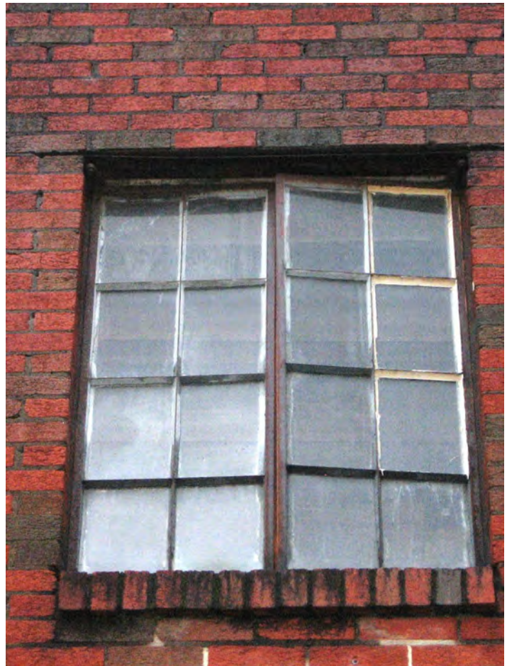
Several buildings in the downtown area retain original steel windows which are an important part of their original design. (116 N. White Street).
