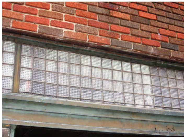
Do not conceal or cover original storefront features like this multi-light glass transom at 11 N. Jackson Street.
