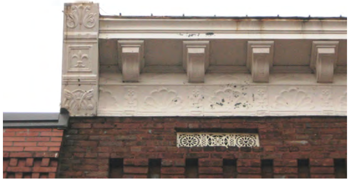
This original sheet metal cornice at 5 W. Washington Avenue is well maintained and is a major feature of this commercial building.
