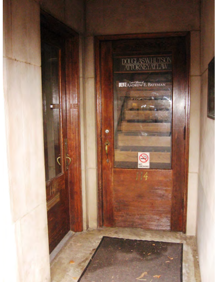
The building at 114 E. Washington Avenue has an original single-light glass and wood door.
