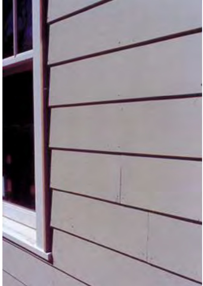
Cementitious siding may be appropriate for new construction, repairs on garages, and repairs on the rear elevations of dwellings.
